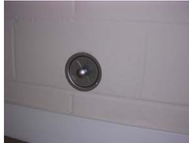
Air vent closed
